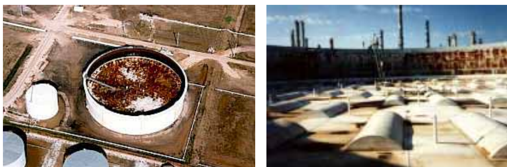
Figure 2.5 - Picture of a floating roof tank.
